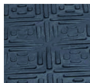
Standard non-skid surface
